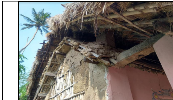
Fig 1: A disaster risk resilient building in the villages of Coastal Odisha (Attu with Thatching)
