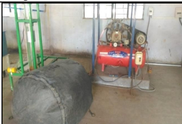
Fig. 11 Raw biogas compression and storage
